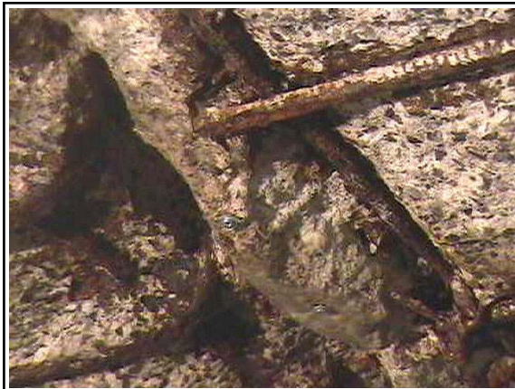
Fig. 3. A close-up view showing the extent of damage and the rusted rebars at one of the locations of the ceiling.
