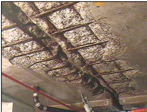
Fig. 11. Typical appearance of the sound concrete and rust-free rebar achieved with the nonrotating single-orifice waterjet.
