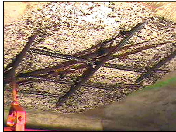
Fig. 10. Typical appearance of the sound concrete and rust-free rebar achieved with the twin-orifice rotating waterjet.
