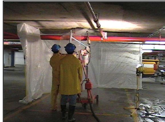
Fig. 6. A general view of the work in progress showing (a) barricades (polythene sheets) set up to protect the pipes carrying compressed air, electrical components, sprinklers, etc.
