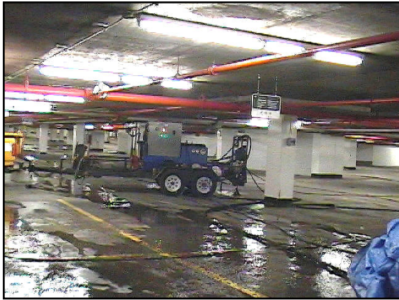
Fig. 5. A general view of the lower-level parking garage of the government building in Ottawa, Canada. The network of pipes on the ceiling must be noticed. Trailer mounted pump was located away from the work area.
